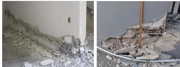
Fig. 2 Flexure failure through concrete crushing and bar buckling/fracture: (a) the 2010 Chile earthquake and (b) 2011 Christchurch earthquake
