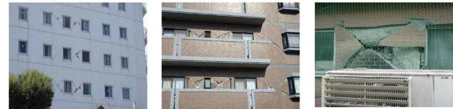
Fig: Damage to NS walls in past earthquakes
