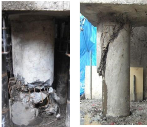
Fig.1: Damage to precast piles during 2016 Kumamoto Earthquake (photo courtesy : Prof. Osamu Kaneko)
