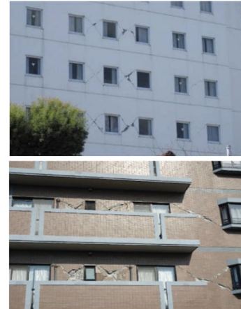
Fig: Damage to NS walls in past earthquakes
